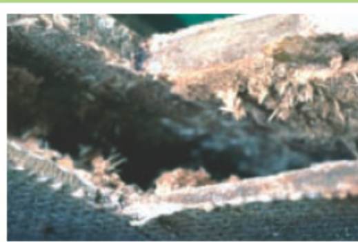
The corner cross-sectional view of a hatch opening shows where rotted core has been reamed out for repair, prior to fitting a new hatch.
