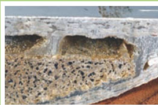
This cross-section of deck laminate shows voids near the outboard edge of the deck where core ends and solid laminate begins.
