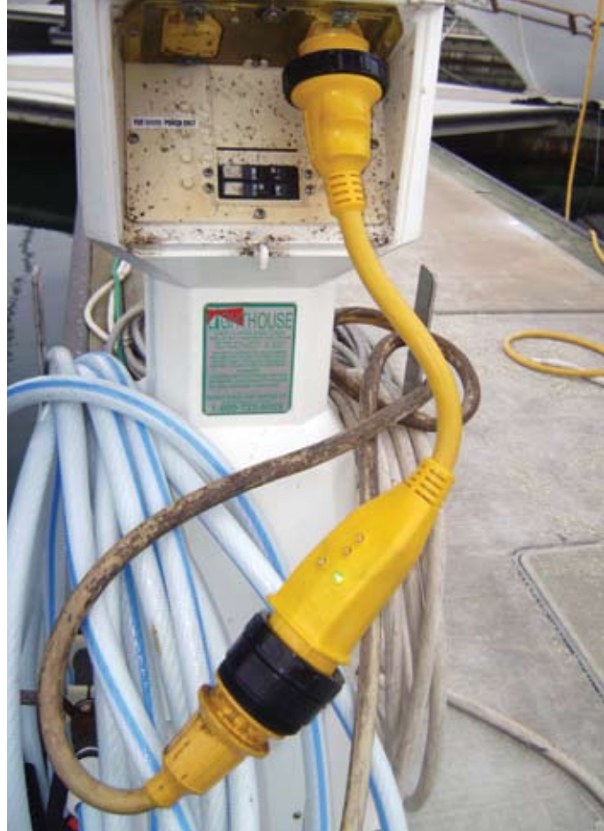
The GalvanAlert's four lights warn of problems in the shorepower system.
